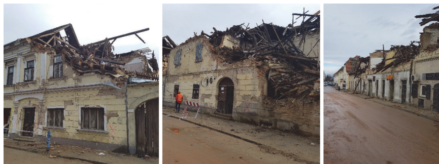
Figure 6. Damage state IV (DS IV) with OOP mechanisms [17]
