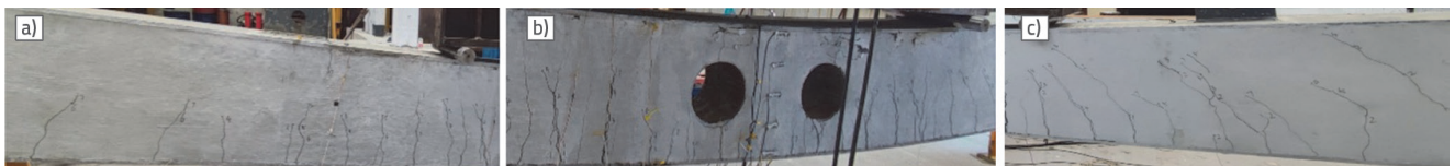
Figure 13. Final failure state of specimen PECB4: a) North side area; b) Mid-span region; c) South side area
