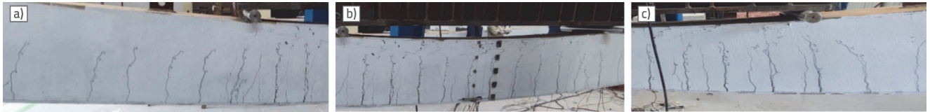
Figure 11. Final failure state of specimen PECB2: a) North side area; b) Mid-span region; c) South side area
