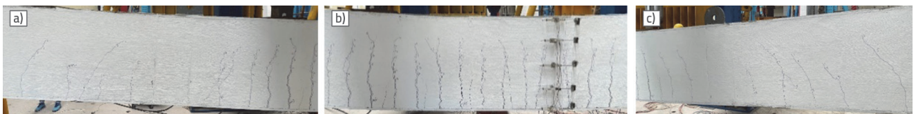
Figure 14. Final failure state of specimen PECB5: a) North side area; b) Mid-span region; c) South side area
