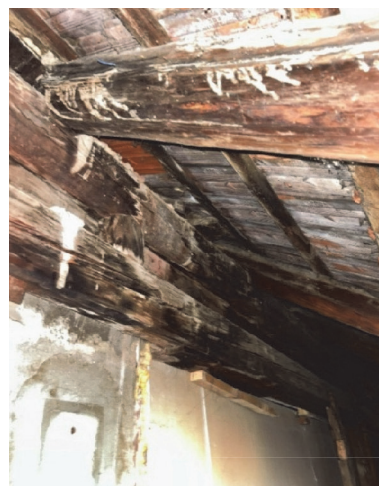
Figure 4. Timber structure damaged by biological agents
