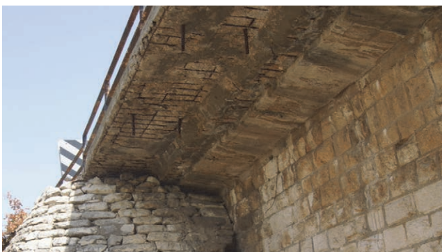
Figure 5. Poor condition of bridge cantilevers
